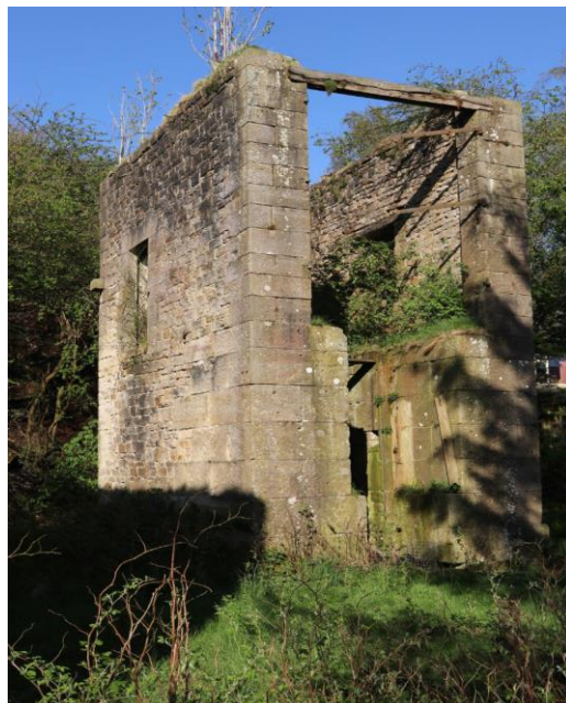
One of only two intact Bull Engine Houses in England at Roachburn, Carlisle
